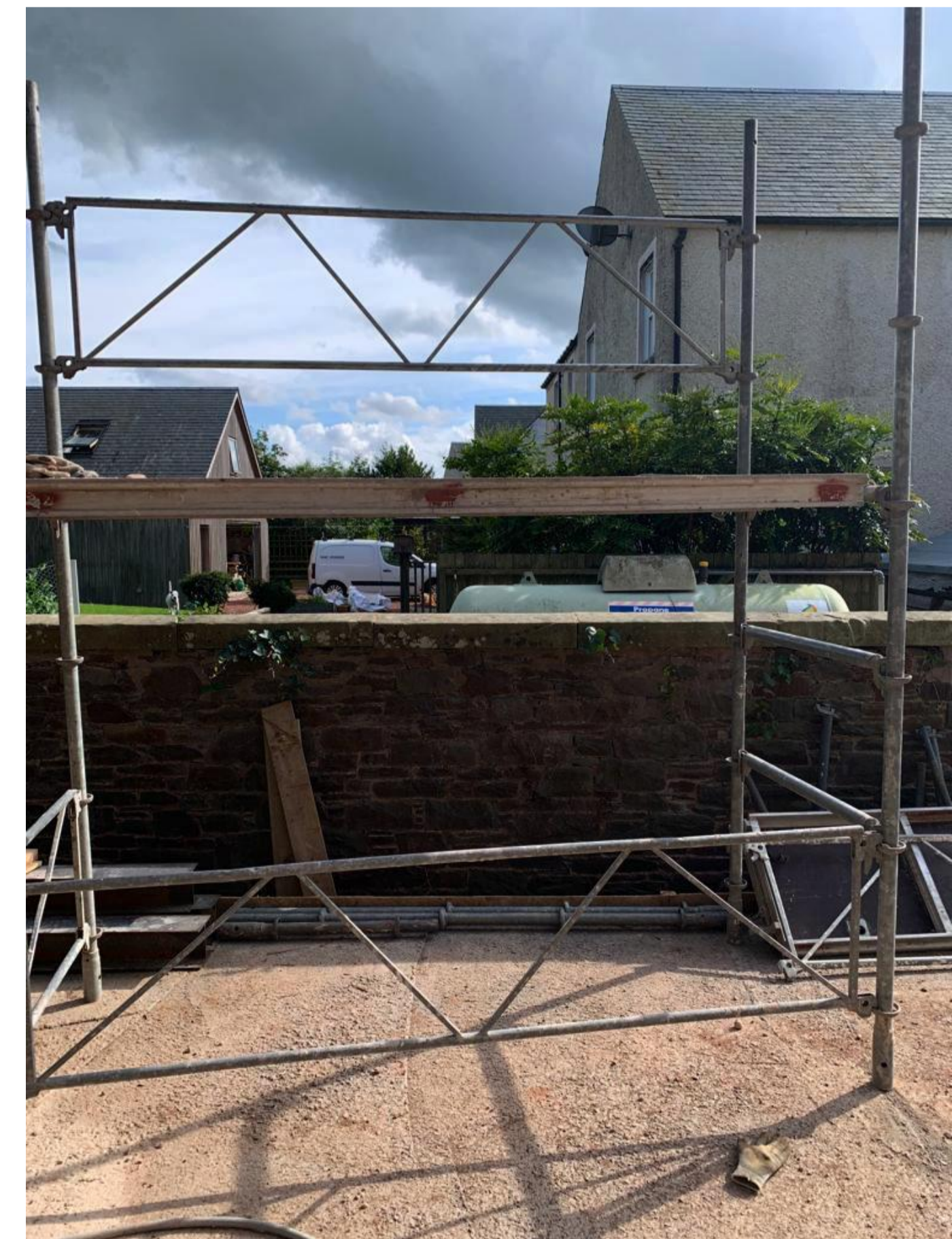
View over boundary wall. Note obstructions - existing gas tank, trees and fencing screen.
